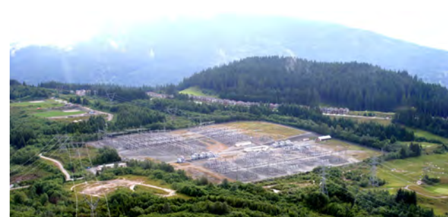
Alternative 2 would run from the Meridian Substation (pictured), in Coquitlam, to the Mount Pleasant Substation in Vancouver.
